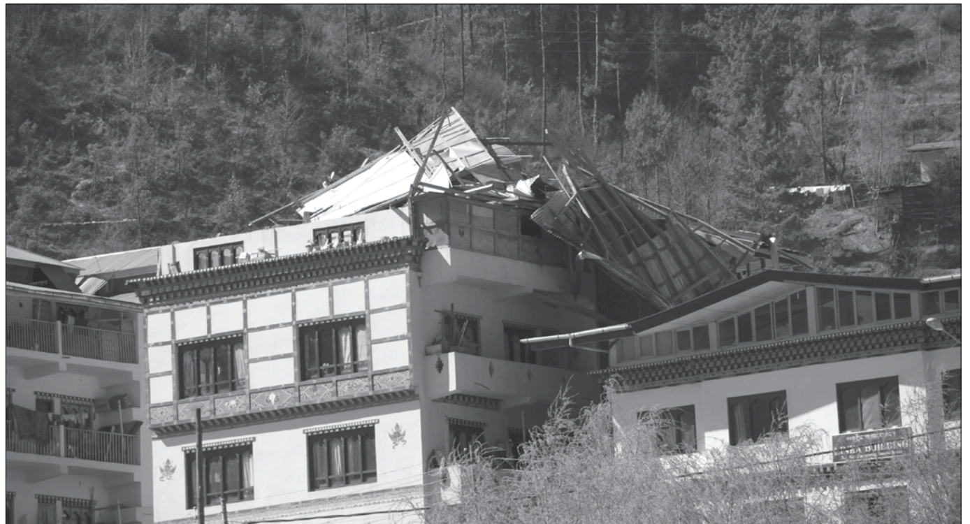
Roof of a building blown off by a windstorm on Wednesday in Changbangdu, Thimphu. Some people were living in the attic of the house. Strong winds that hit several western dzongkhags on March 8 and 9 damaged several homes, lhakhangs, and schools. The scale of damage is yet to be ascertained.
